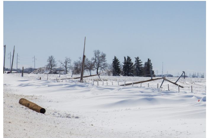
Stay away from downed power lines, but call LEC at 889-3301 to report the situation.
