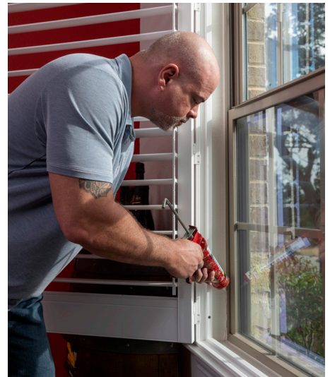
ABOVE: Sealing air leaks around your home is a simple, effective way to save energy and lower your bills.
